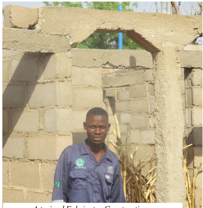
A trained Fabricator Constructing a house and new workshop in Sitti , Sumaila LGA
