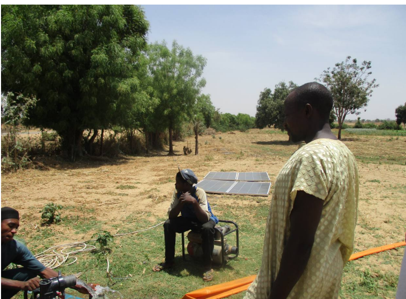
Solar powered pump at Watari in Ungogo LGA
